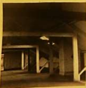
ATTIC OF 1795 TROOP & STABLE BLOCK. AN UNSUITABLE BARRACK ROOM. SEE FIG. 2.
