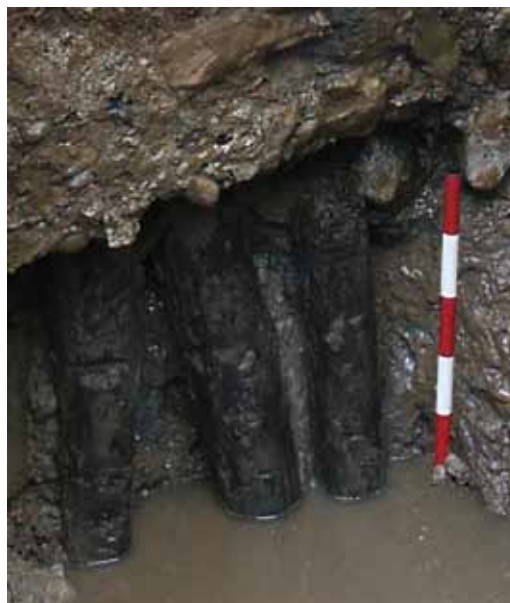
Wooden piles beneath the foundations of the Multangular Tower. (scale intervals: 100mm)
