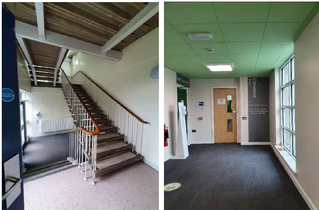
Communal spaces in Derwent Block P – original stairwell and modernised reception lobby leading to the seminar rooms
